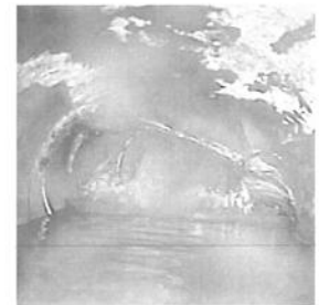
Structural defect and pipe deformation
