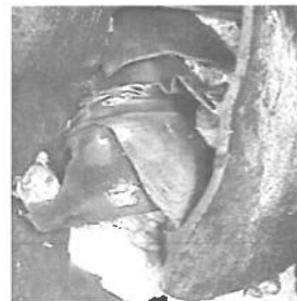
Wastewater pipe failure
