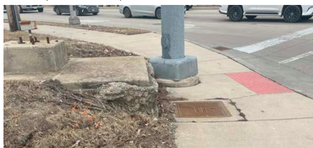
Figure 4. SW Corner. No pedestrian accommodations and non-compliant ADA ramps.
