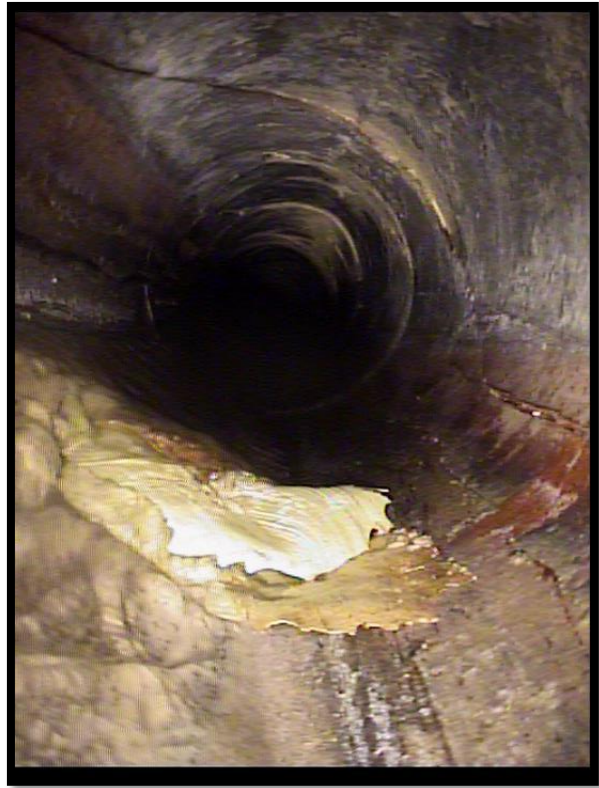
Future Collapse of Pipe
