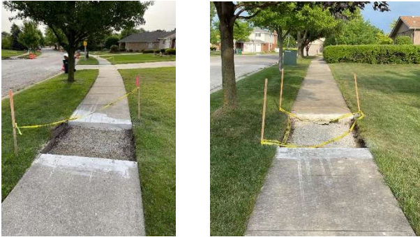
Before: Type II Barriers missing
