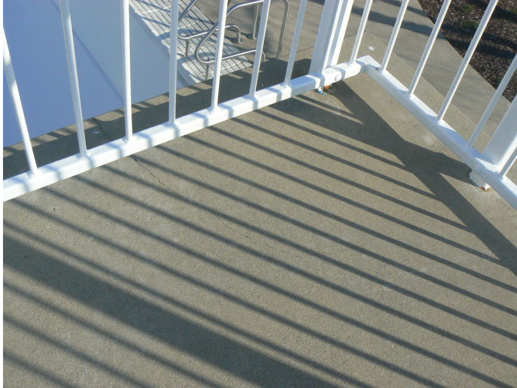
Crack E over top of northeast column
