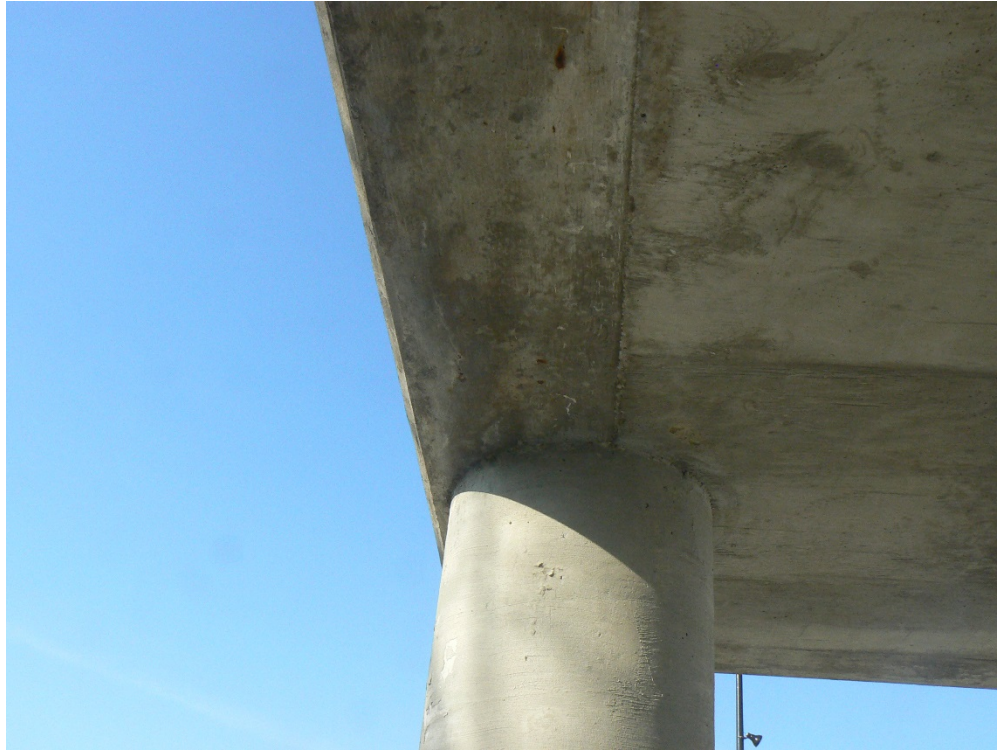
Crack F – Underside of main platform
