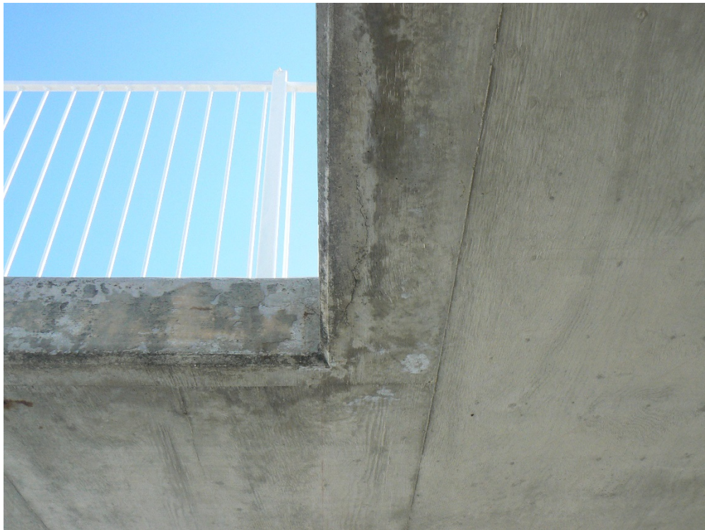
Crack D – Underside of main platform
