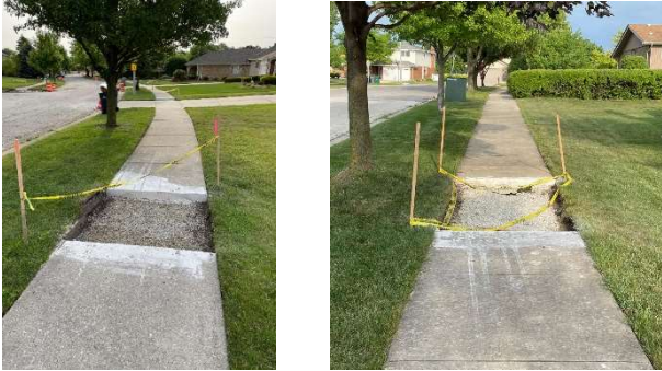
Before: Type II Barriers missing
