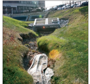
Eroding Channel, Silver Cross Hospital, Joliet
