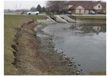
► Eroding banks along basin shoreline
