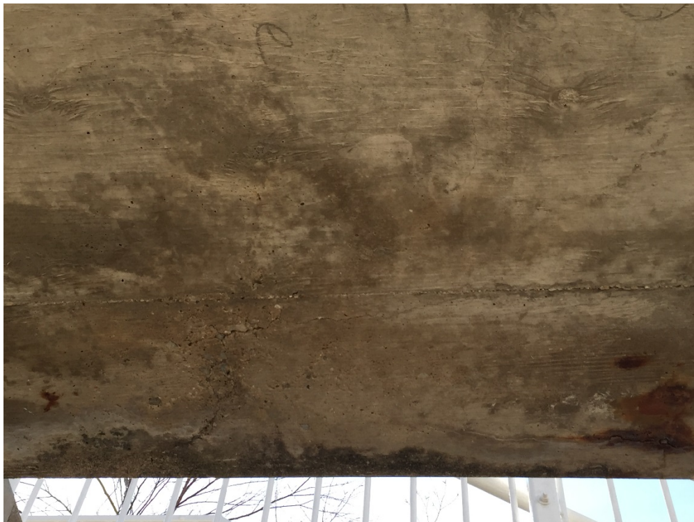
Crack B/H – Underside of main platform
