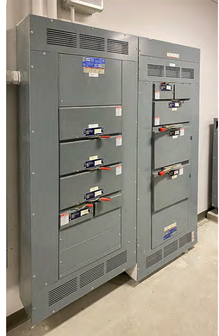
Police Station existing power distribution system
