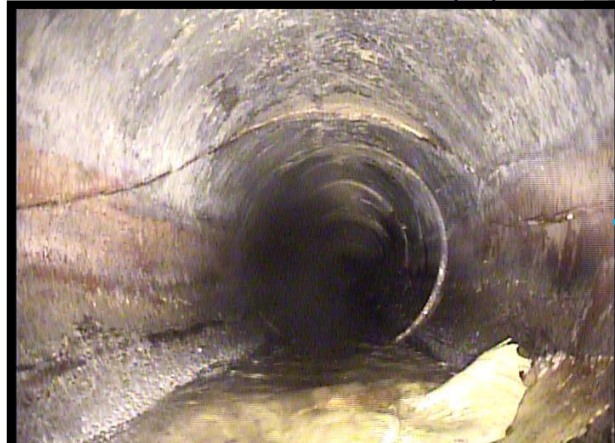
Crack in pipe
