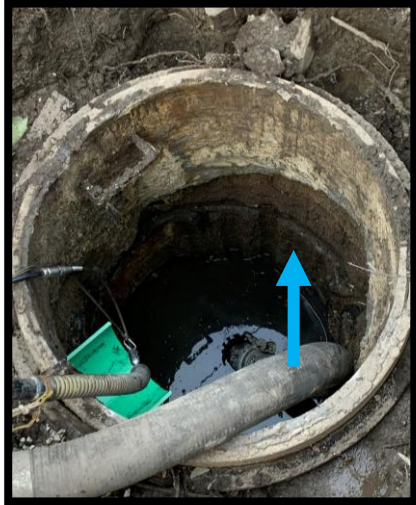
Concrete missing in manhole
