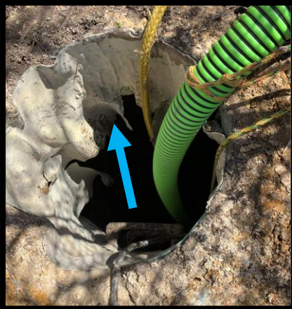
Liner peeling away from structure
