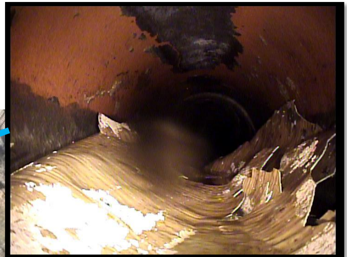
Previous 2004 repairs of epoxy resin liner of manholes in pipe
