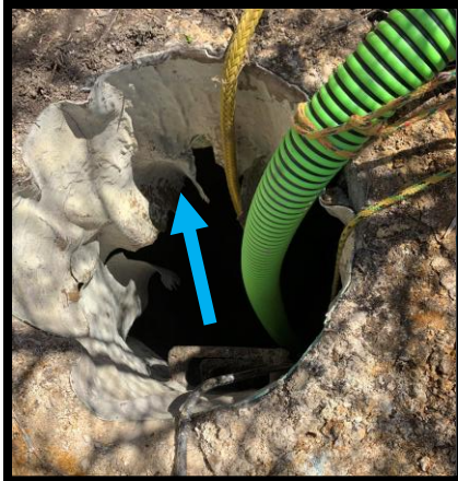
Liner peeling away from structure
