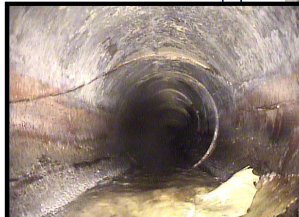
Crack in pipe
