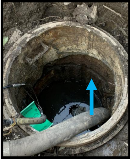
Concrete missing in manhole
