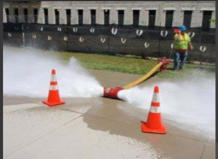
Fire Hydrant Program
