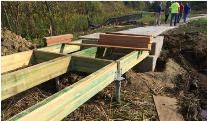
Existing wetlands were traversed with boardwalks utilizing helical piers to limit wetland disturbance.
