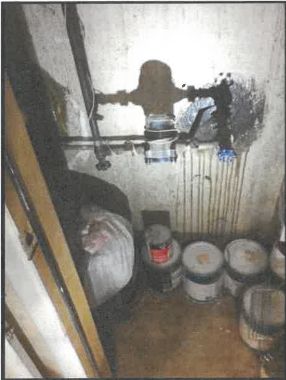
Pre Installation Photo
