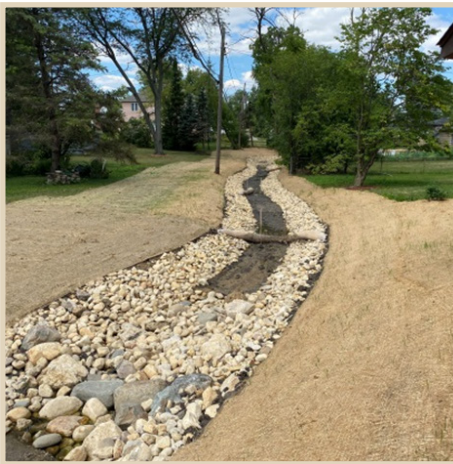
St. Joseph Creek design/build project for Downers Grove included native vegetation slope with rip rap toe.
