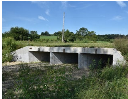
Box culvert was designed to better align with the stream to improve hydraulic and scour conditions.
