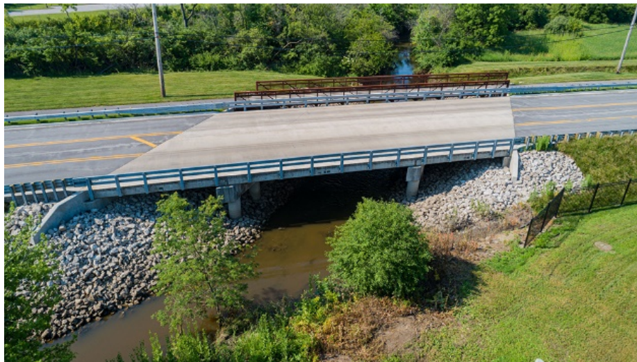
Three-span PPC deck beam bridge and pedestrian bridge over Union Creek in Frankfort, IL.
