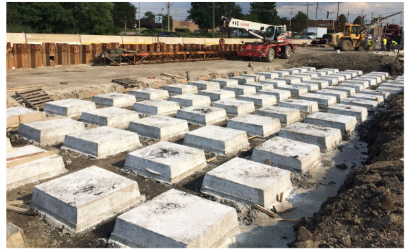
Prior to a dryland bridge design, a preliminary support system study will be performed to identify cost-effective solutions.
