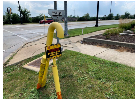
We have experience designing around petroleum pipelines.
