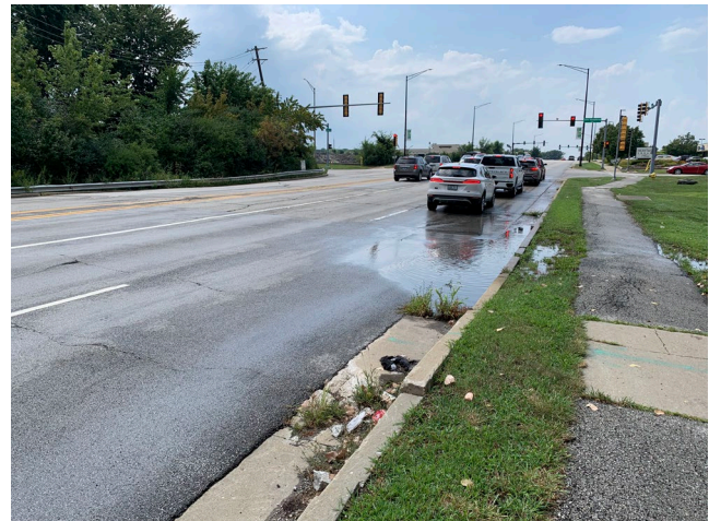
A new dryland bridge will be constructed on the east leg of the intersection where settlement is obviously occurring.
