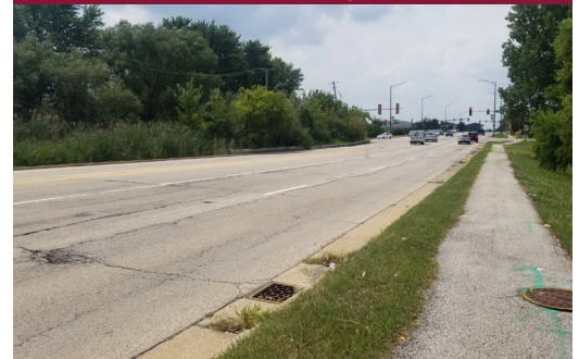
Settled Pavement along 143 rd Street
