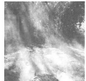
Multiple manhole I/I sources found during smoke testing
