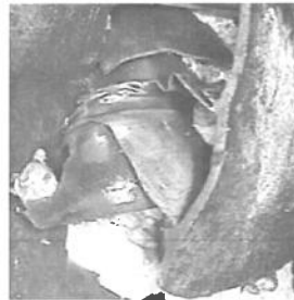
Wastewater pipe failure
