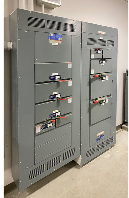
Police Station existing power distribution system
