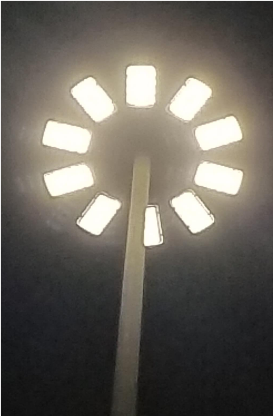
New LED Luminaires
