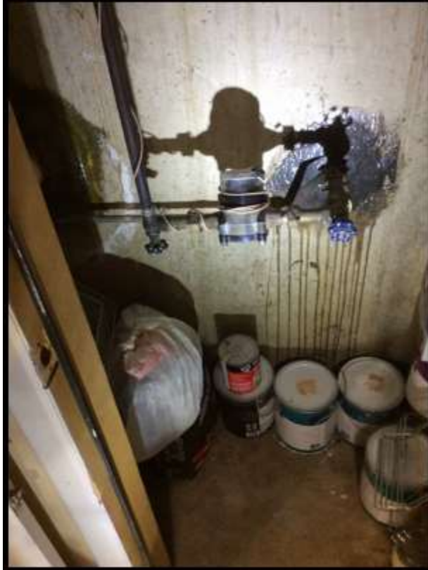
Pre Installation Photo
