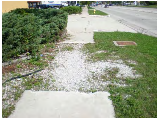
Missing sidewalk on west side of La Grange Road near 144 th Street
