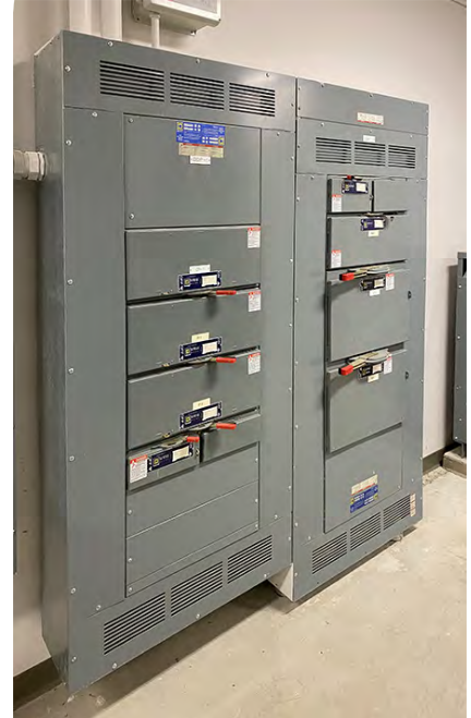
Police Station existing power distribution system
