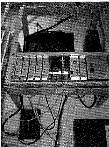
Under view of rack system in closet
