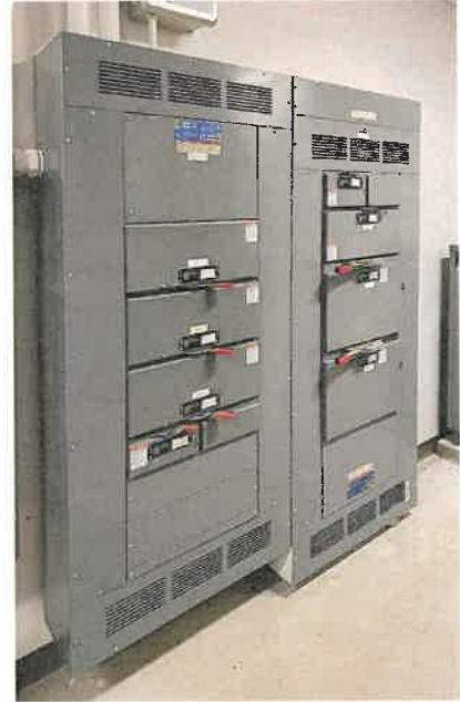
Police Station existing power distribution system
