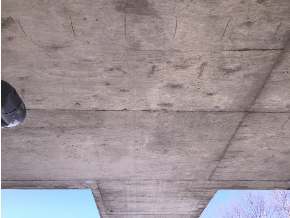
Crack B - Underside of main platform
