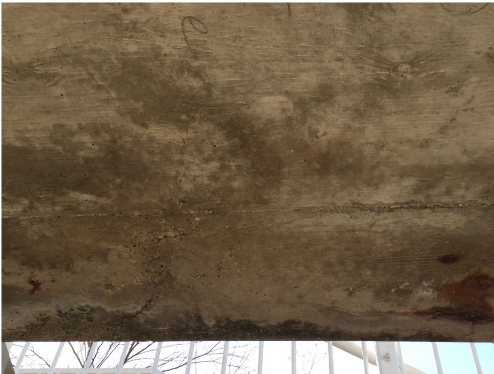
Crack B/H – Underside of main platform
