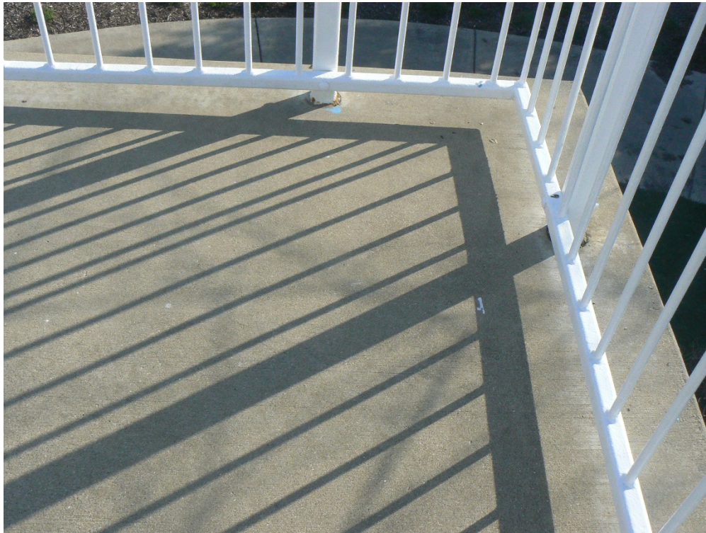
Crack G on top slab over southeast corner
