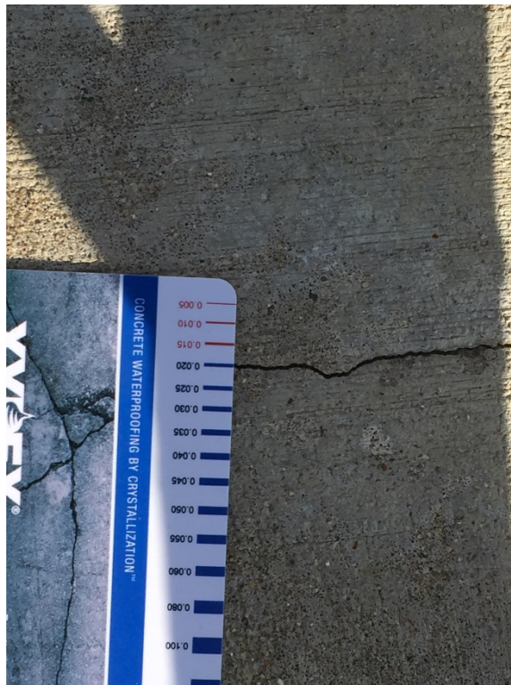
Close-up of crack A on top slab – measured 0.020"
