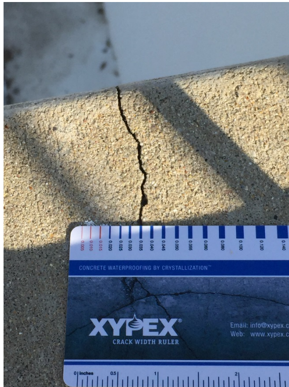
Close-up of crack E on top slab – measured 0.035"
