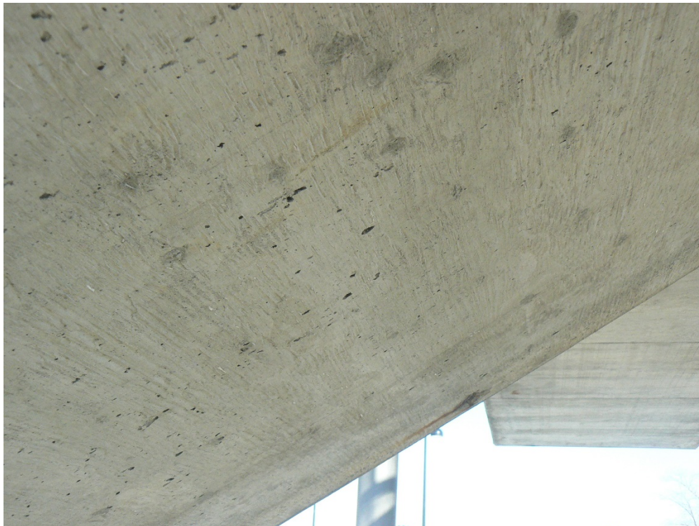
Crack I - underside of stairs – hairline crack, probably too small to inject at this time
