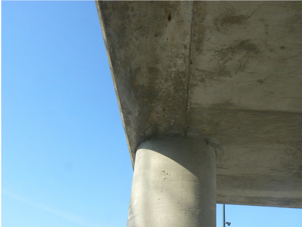
Crack F – Underside of main platform
