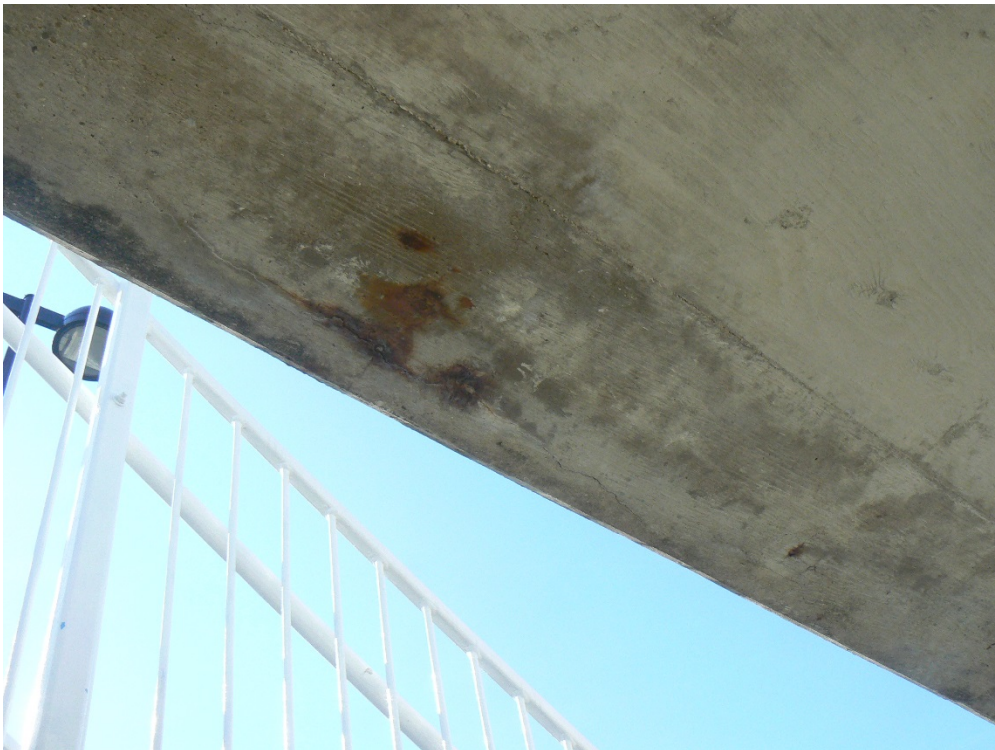
Crack G – Underside of main platform – with minor rust and efflorescence
