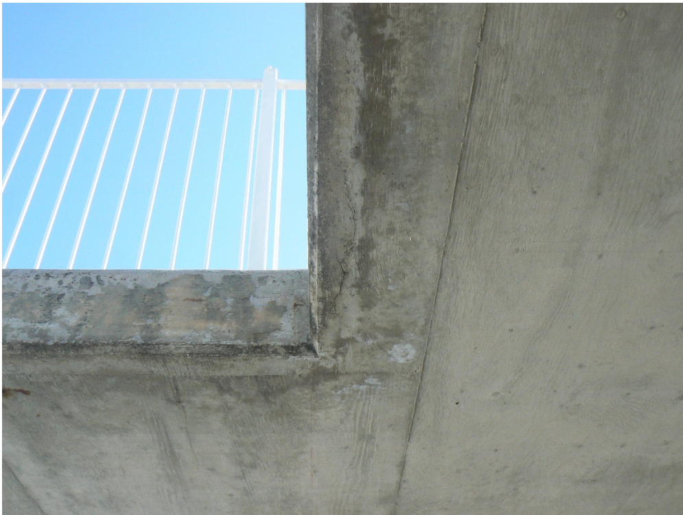
Crack D – Underside of main platform
