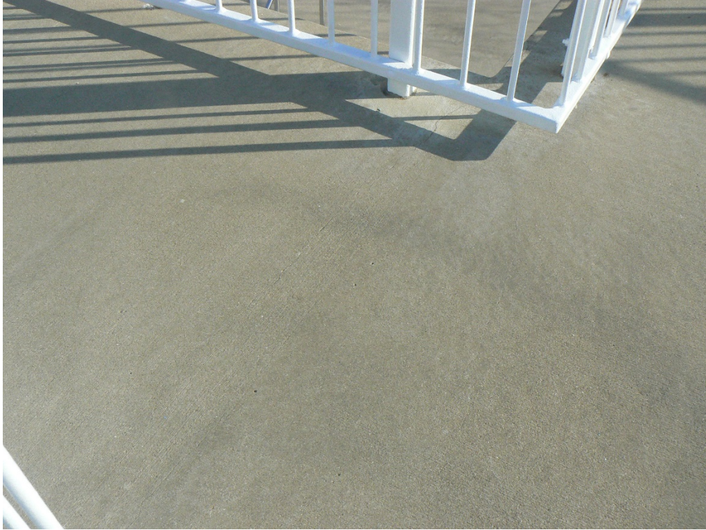
Cracks A-D on top slab – located at edge of diving platform
