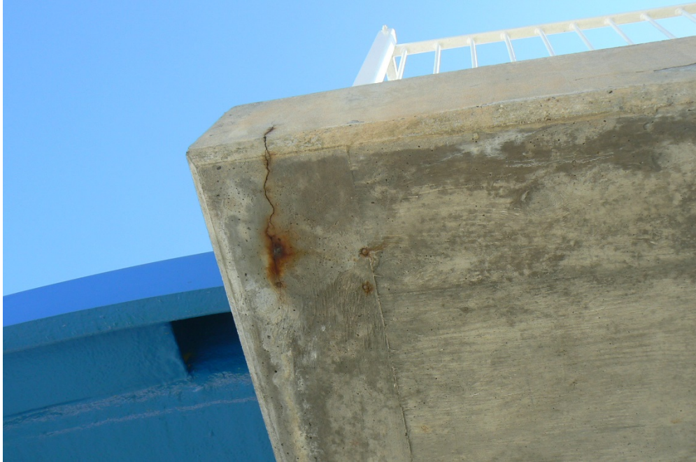
Crack E - Underside of main platform – northwest corner
