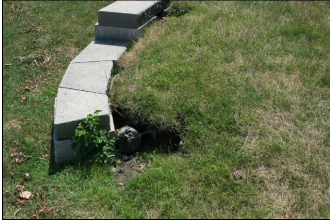
Stormwater runoff has eroded the land around this retaining wall. Photo courtesy of Beth Corrigan
