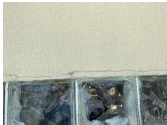
Large crack across the top of the window
