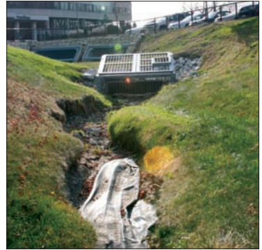
Eroding Channel, Silver Cross Hospital, Joliet
