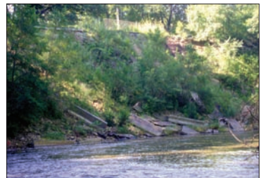
Severe erosion threatening roadway, Hickory Creek at Hillcrest Road
